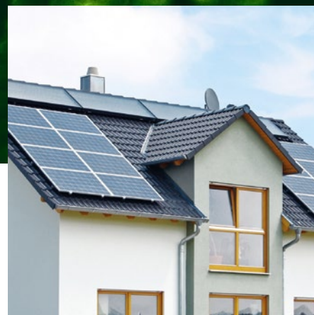
PHOTOVOLTAIC MODULES AND INVERTERS
